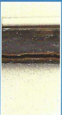
Split Vertical Pipe in Interior Walls
