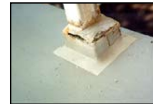
Rail post degradation
