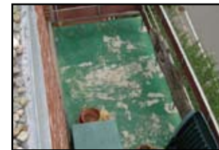
Failed balcony coating
