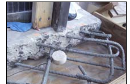
XP+ Anodes used to prevent corrosion of rebar near the balcony edge
