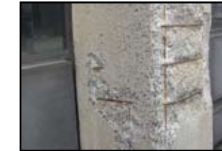
Poor concrete cover
