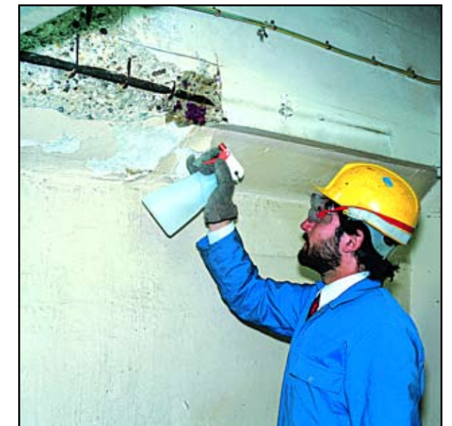
Testing to identify carbonated concrete. Purple indicates a high pH while no color change signifies carbonated concrete
