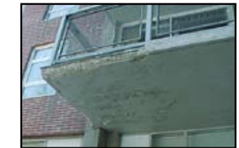
Underside balcony spalls
