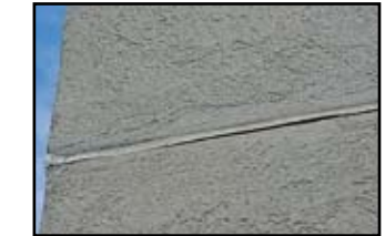
Sealant adhesion failure
