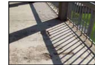
Balcony surface erosion
