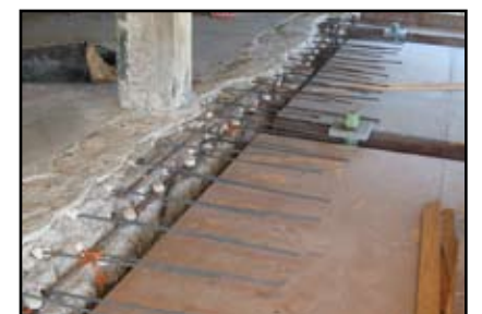
XP+ anodes installed where an existing slab and a new, full-depth slab meet
