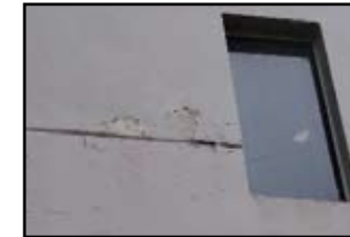
Failed facade coating
